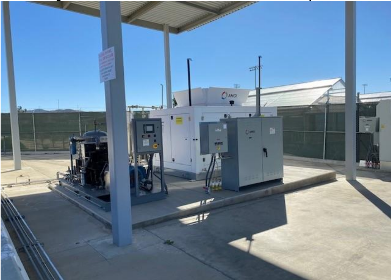
Figure 1: Lake Elsinore Unified School District CNG Compressor
