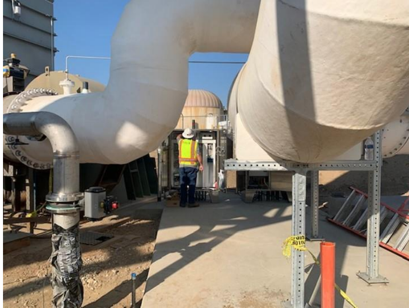
Figure 12: Commissioning of RTO System for Tail Gas Treatment
