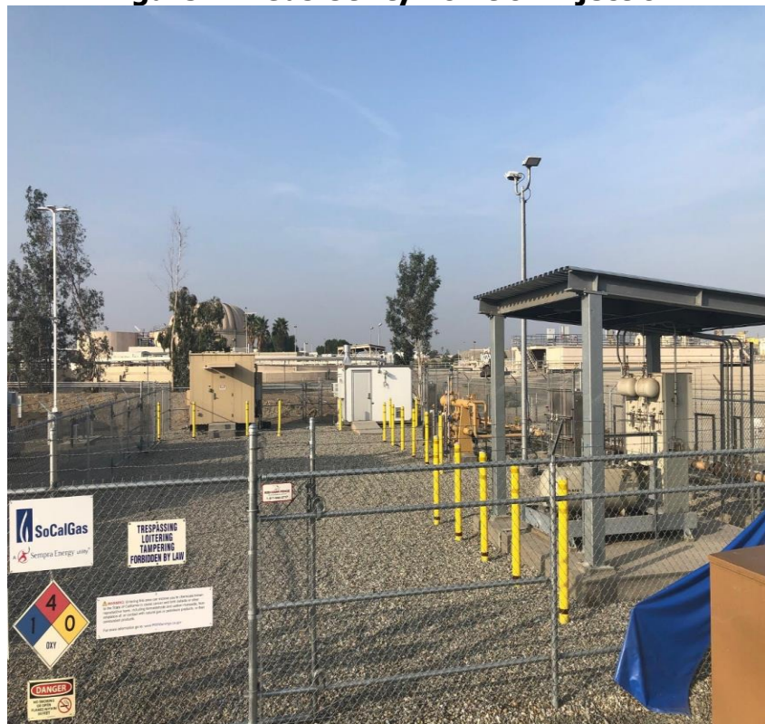
Figure 17: Gas Utility Point of Injection
