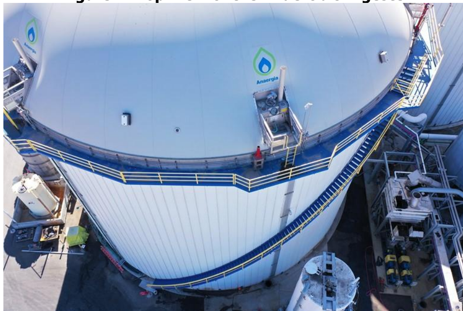
Figure 2: Top View of the Anaerobic Digester
