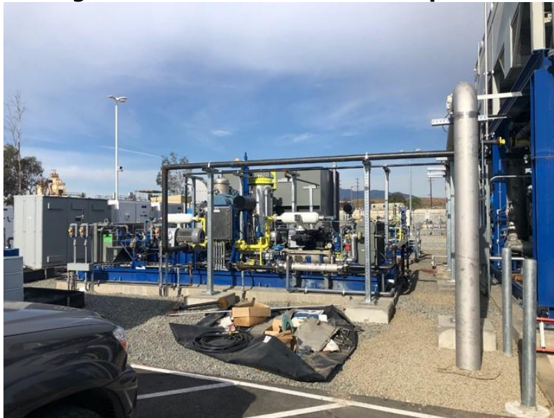
Figure 9: Third Train Product Compressor
