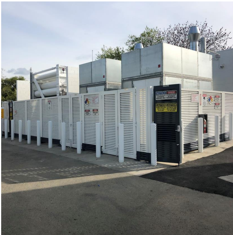
View of the dispensers and POS (above) and fenced equipment compound (below).
