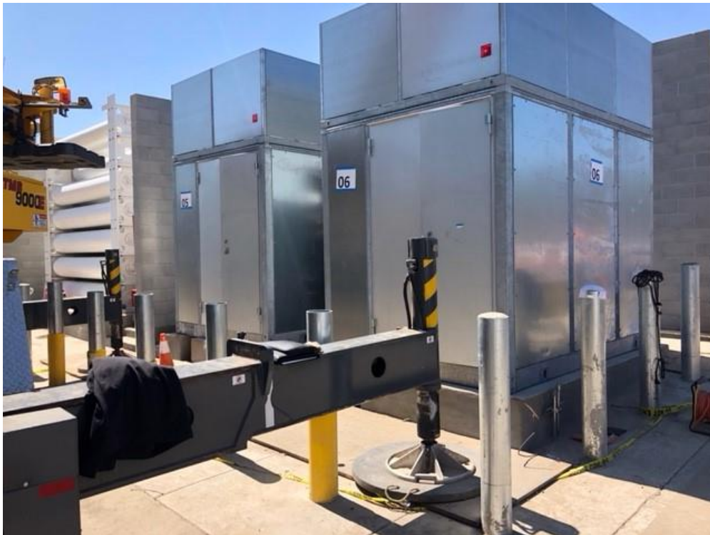
Field assembly of storage module (above) and two compressor modules (below). Photo Credit: Fiedler Group/Shell
