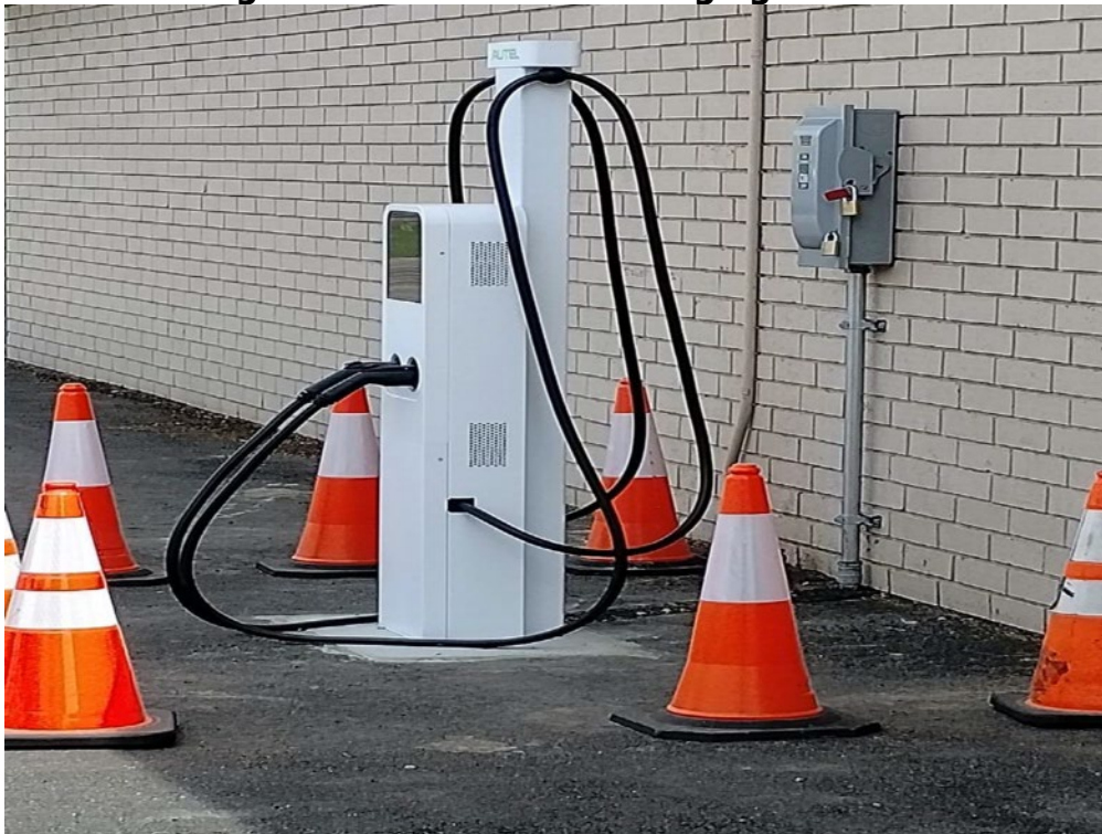
Dual-port EV charging station installed at Calexico High School.
