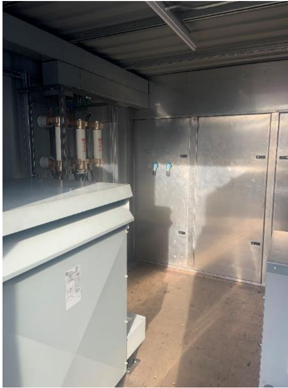
Figure 22 - Interior View of Battery Pack
