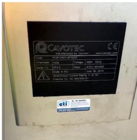
Figure 15 - ETI Verification Sticker Adhered to Cavotec SPS Unit
