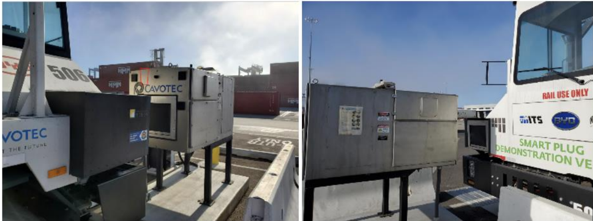
Figure 5 - Cavotec SPS & BYD 8Y Yard Tractor Fully Integrated and Operational
