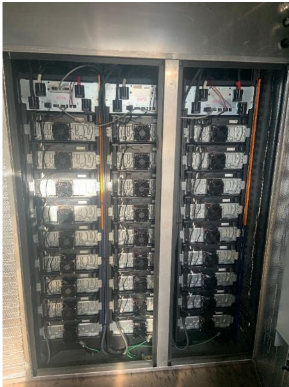
Figure 23 - Rack of Individual Batteries
