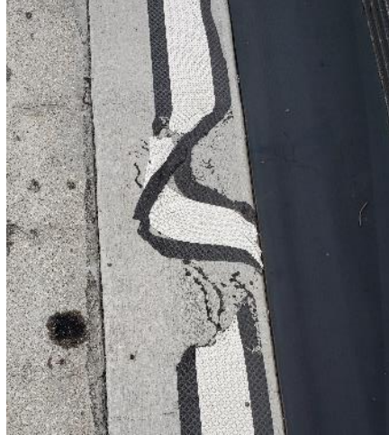
Figure 8 - Damaged Alignment Tape
