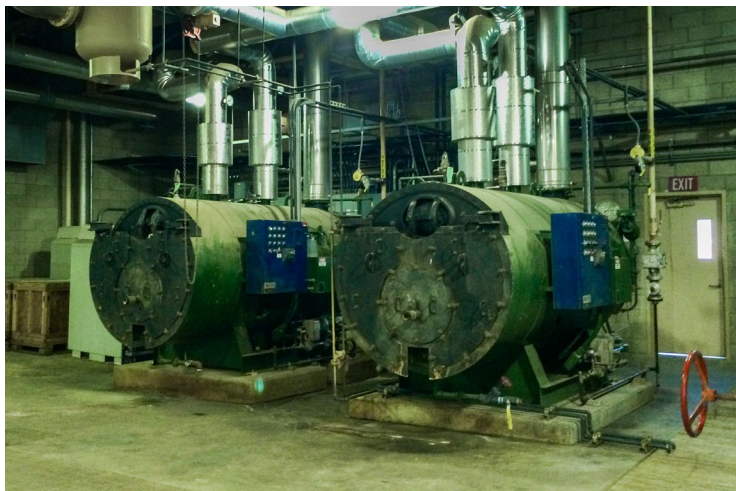
Figure 9: The Two Johnston Boilers at CWRP
