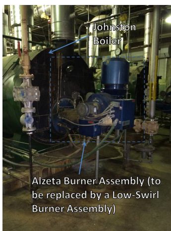
Figure 10: Alzeta Burner Installed at CWRP Boilers
