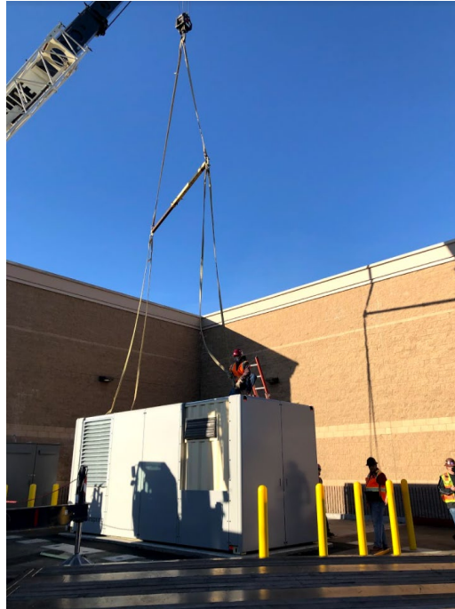
Figure 15: Product Installed at Customer Site Without All Panels
