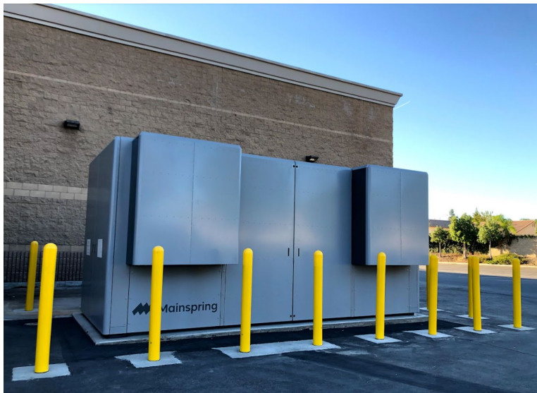
Figure 16: Product Installed at Customer Site With All Panels
