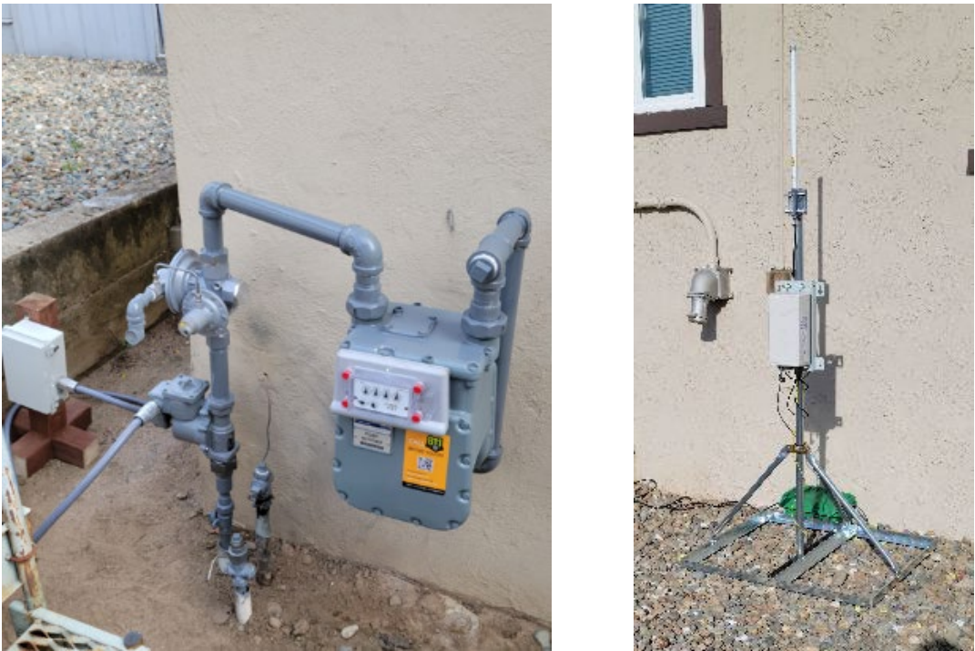
Figure 17: PG&E Commercial Building: (Left) Smart Valve, (Right) Gateway/Antenna Installation
