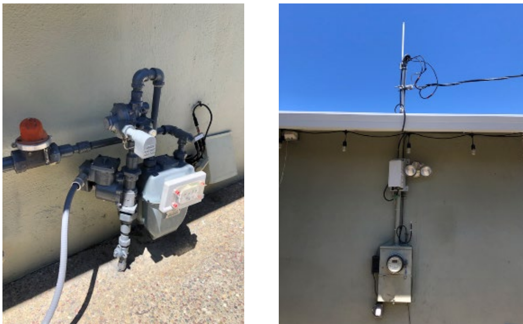
Figure 13: PG&E Residential Building: (Left) Lorax Systems Valve, (Right) Antenna/Gateway
