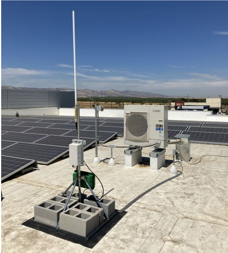
Figure 5: Temporary LoRaWAN® Tektelic Gateway and Antenna Setup
