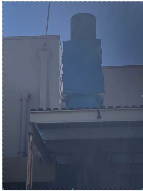
Figure B-18: Porterville Unilux New Boiler Economizer1
