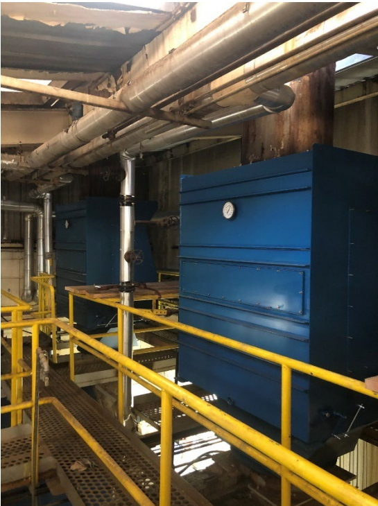
Figure B-15: Livingston Boilers #1 & #2 New Economizers
