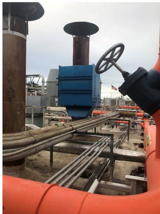
Figure B-12: Turlock FTP1 New Economizer2
