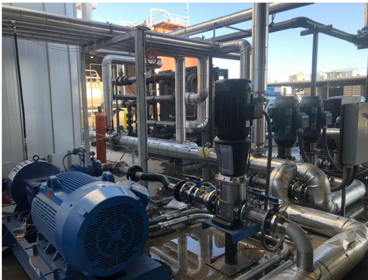
Figure B-7: Pumps
