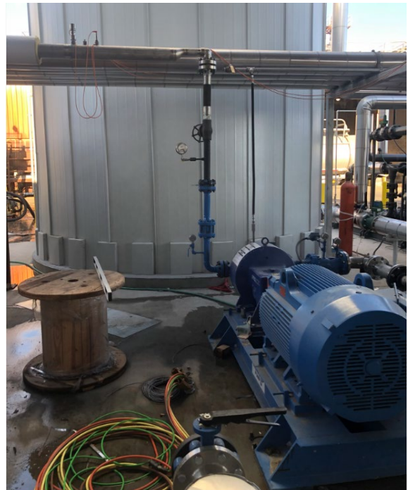
Figure B-8: Pump and Tank
