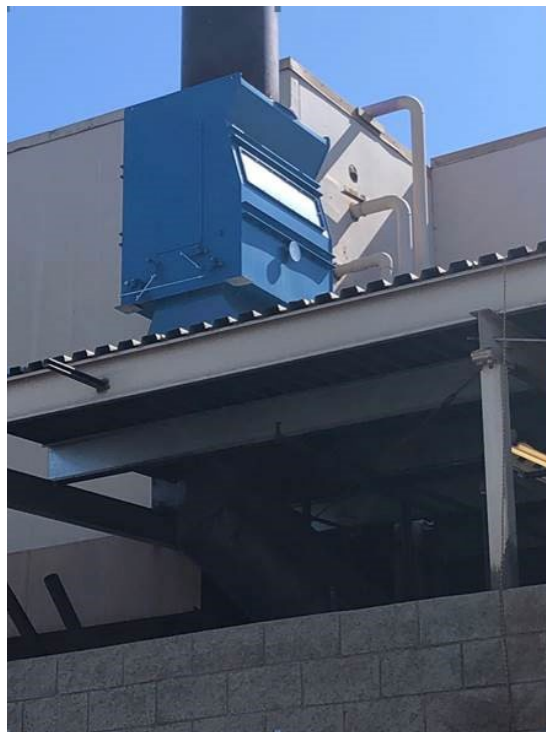
Figure B-19: Porterville Unilux New Boiler Economizer2
