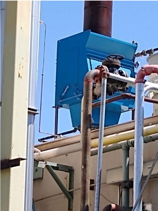
Figure B-13: Fresno Belgravia Boiler New Economizer
