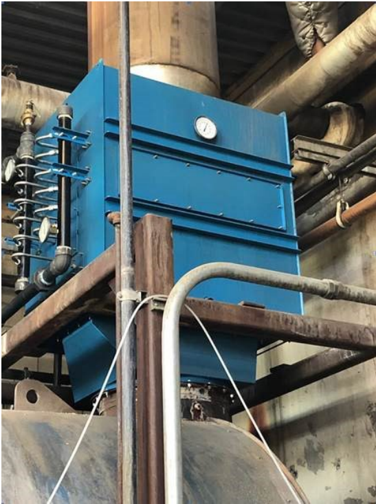
Figure B-17: Porterville Hurst New Boiler Economizer2
