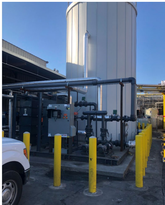
Figure B-10: Control Equipment and Tank
