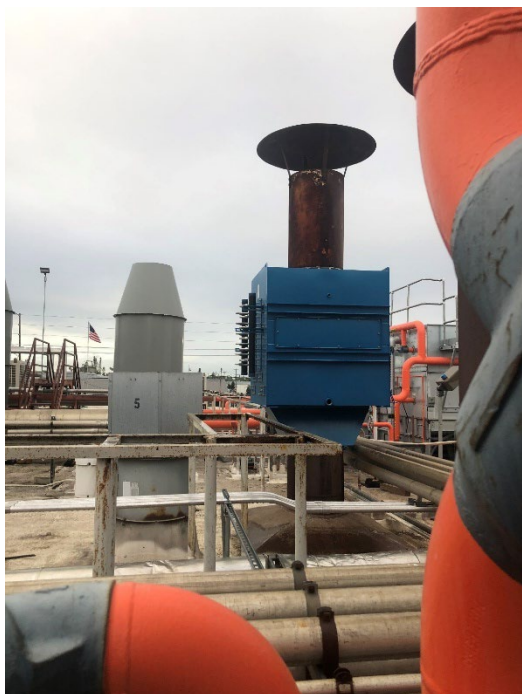
Figure B-11: Turlock FTP1 New Economizer1
