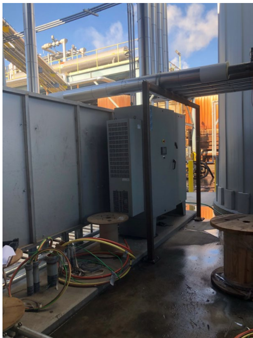
Figure B-9: Electrical Panel
