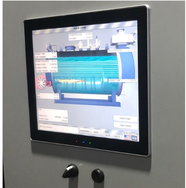
Figure B-2: Livingston Boiler #2 Controls
