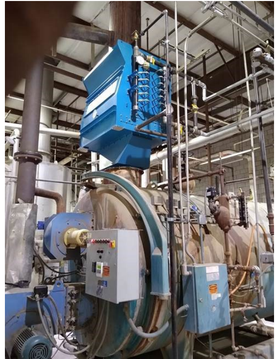
Figure B-14: Fresno Cherry New Boiler Economizer
