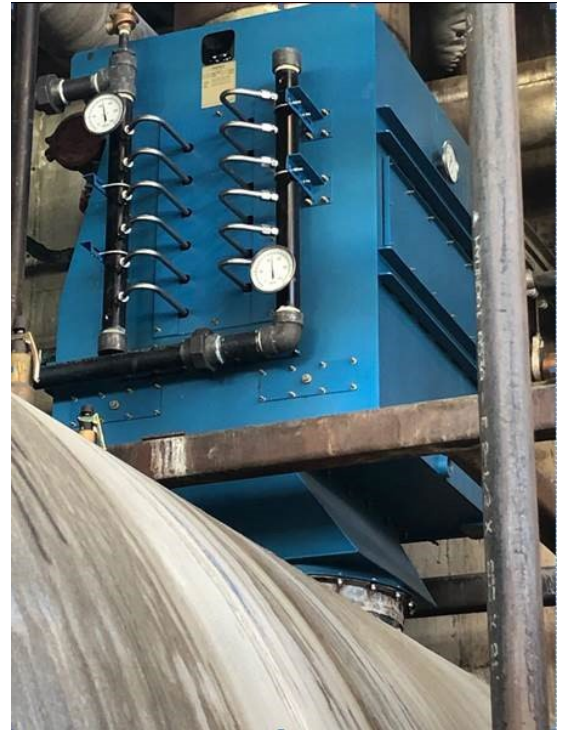
Figure B-16: Porterville Hurst New Boiler Economizer1
