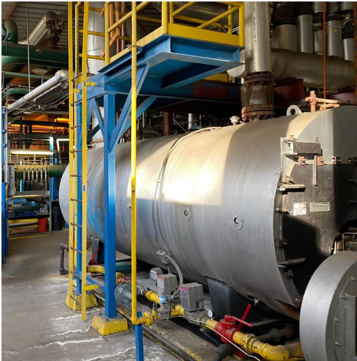
Figure 1: Boiler at DFA's Facility
