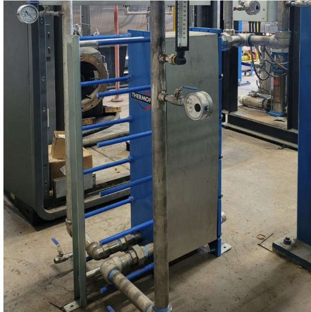
Figure 6: Plate and Frame Heat Exchanger
