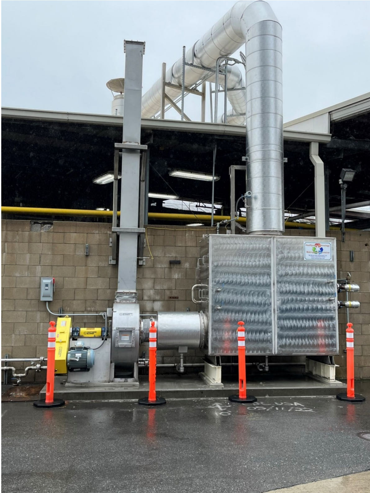
Figure C-4: Installed Fan and HeatSponge Economizer Unit
