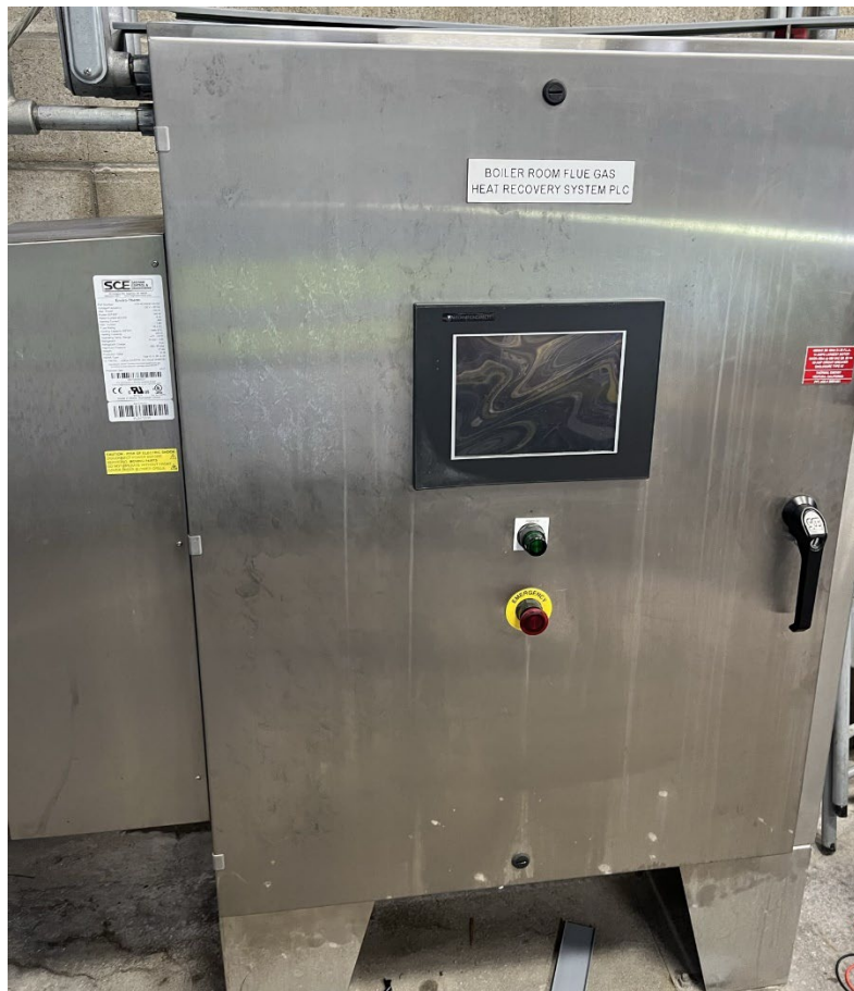
Figure 8: Boiler Room Flue Gas Heat Recovery System Programmable Logic Controller
