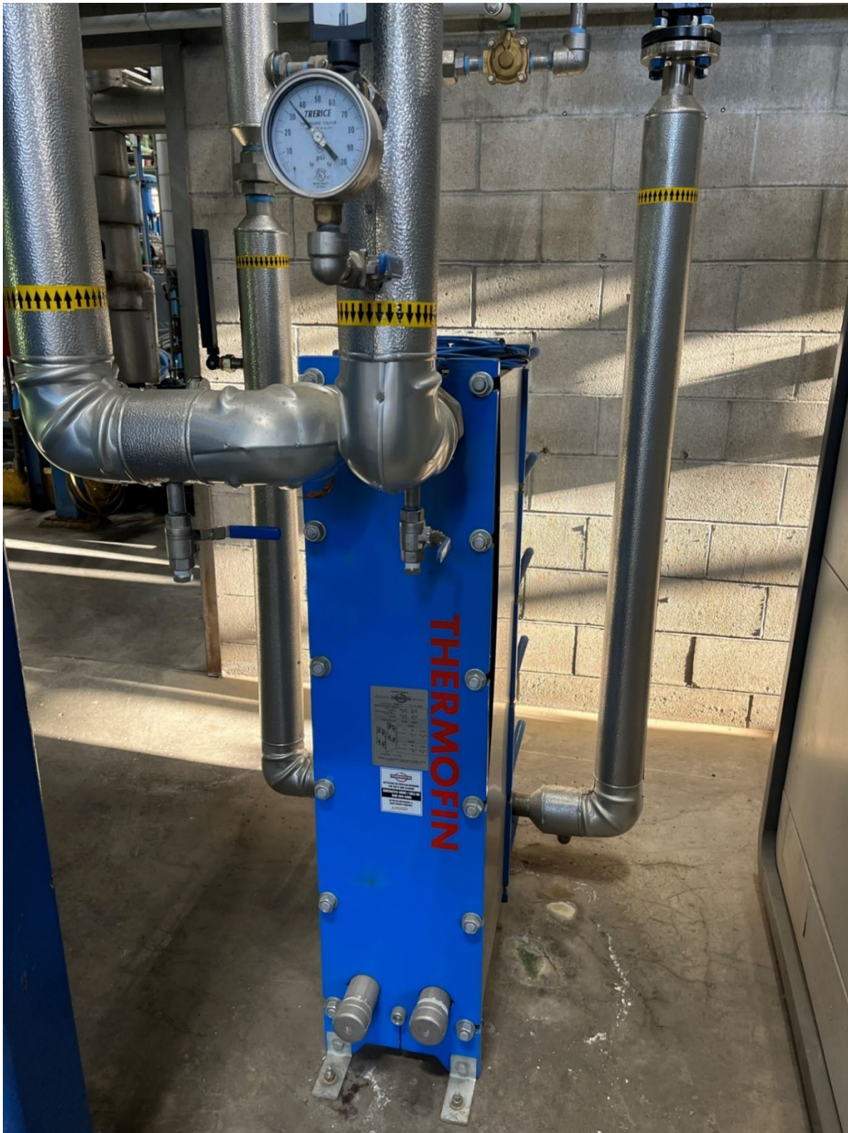
Figure C-5: Installed Heat Exchanger
