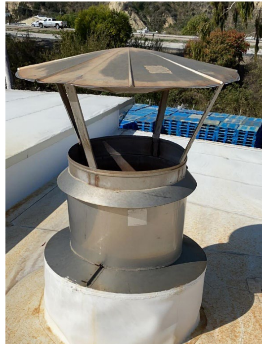
Figure 2: Boiler Exhaust at DFA Facility
