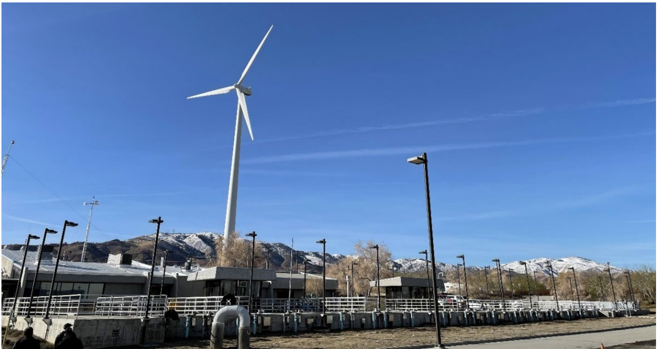
Figure 2: Palmdale Water District's Existing Wind Turbine Generator
