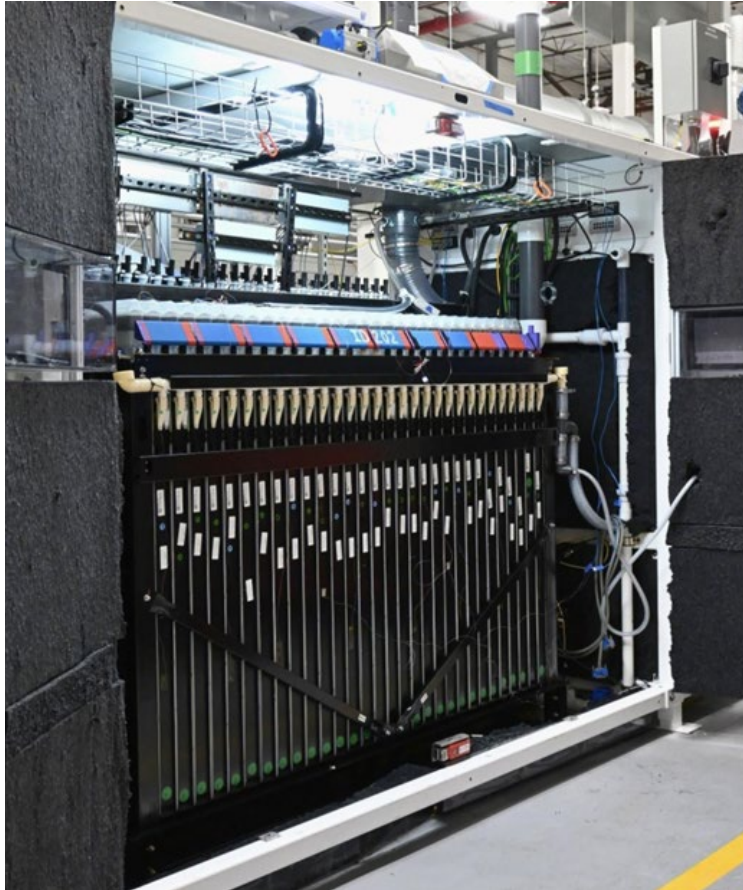
Figure 5: Test Module in its Test Stand in Form Energy's Berkeley Facility
