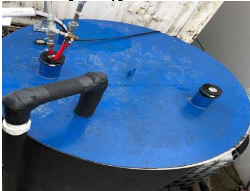
Figure 6: Upgraded Steel Lid
