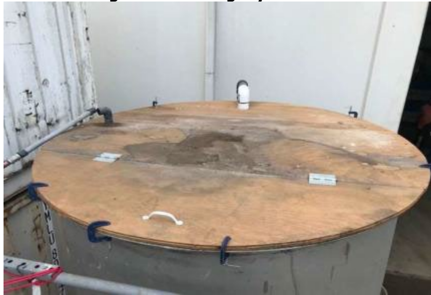
Figure 5: Existing Plywood Lid
