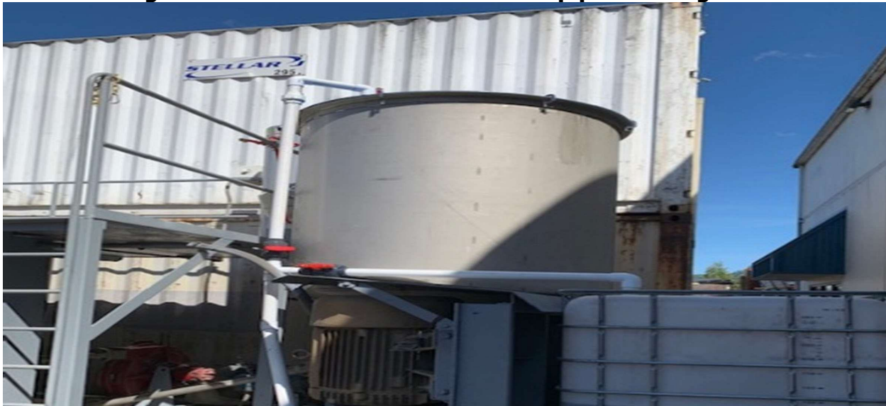
Figure 4: Feed Tanks and Routed PVC pipe to 750-gallon
