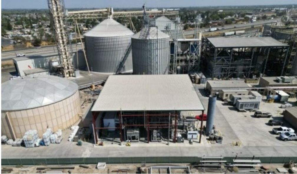
Figure 3: Aemetis Advanced Fuels Keyes Facility with Biogas Upgrading Facility Completed Under Overhang
