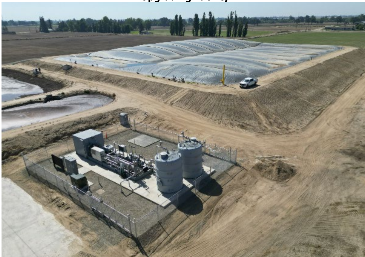
Figure 15: Dairy that transports biogas via pipeline to the Aemetis Biogas Upgrading Facility
