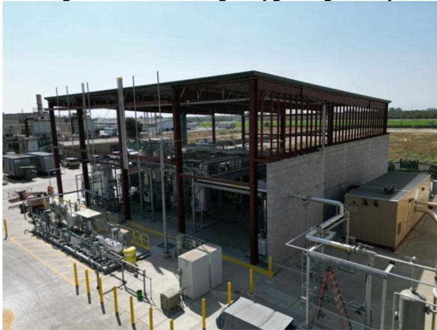
Figure 1: Aemetis Biogas Upgrading Facility
