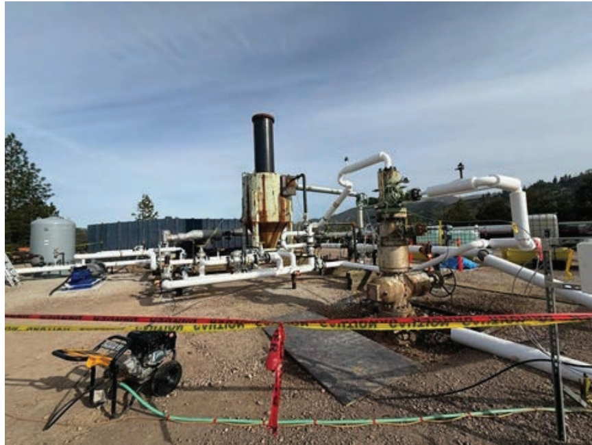
Picture of the well, surface piping system with the silencer visible in the background. The DTS stand can be seen towards the right, close to the wellhead.
