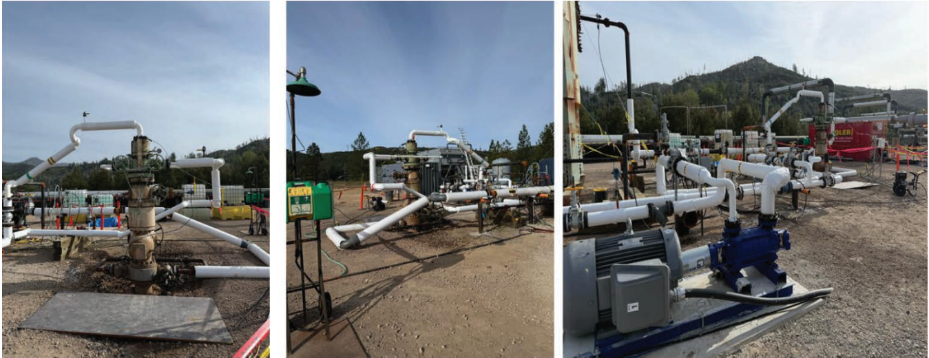
Figure 6: GreenFire’s AGS in Well DV-13 at The Geysers Geothermal Field
