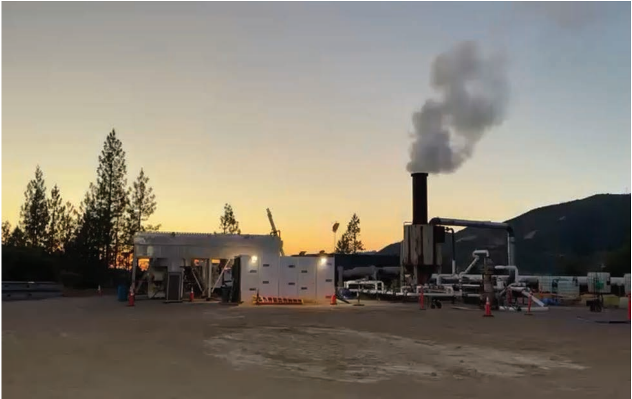
Figure A.8: The Complete Surface System of the AGS Captured during a Forward Flow Operational Mode Test, Demonstrating How the System Releases Excess Steam
