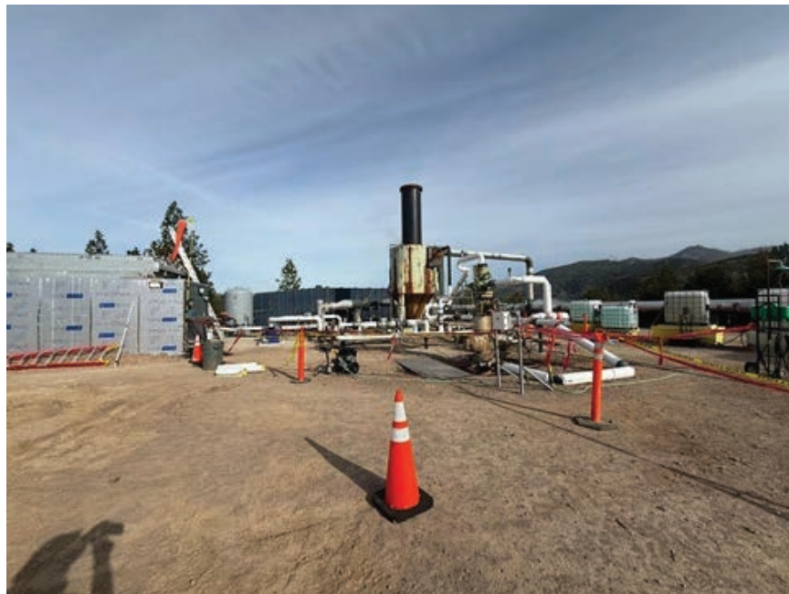
Picture of the surface circulation loop and control units. Chemical containers are also visible on the right side of the picture, used for gas treatment.
