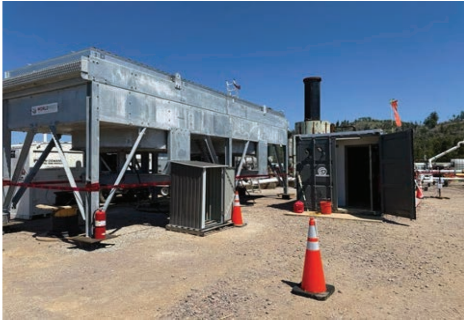
Figure A.6: Picture of the Air Cooler on the Left Side and the Entrance to the AGS Control Unit on the Right Side
