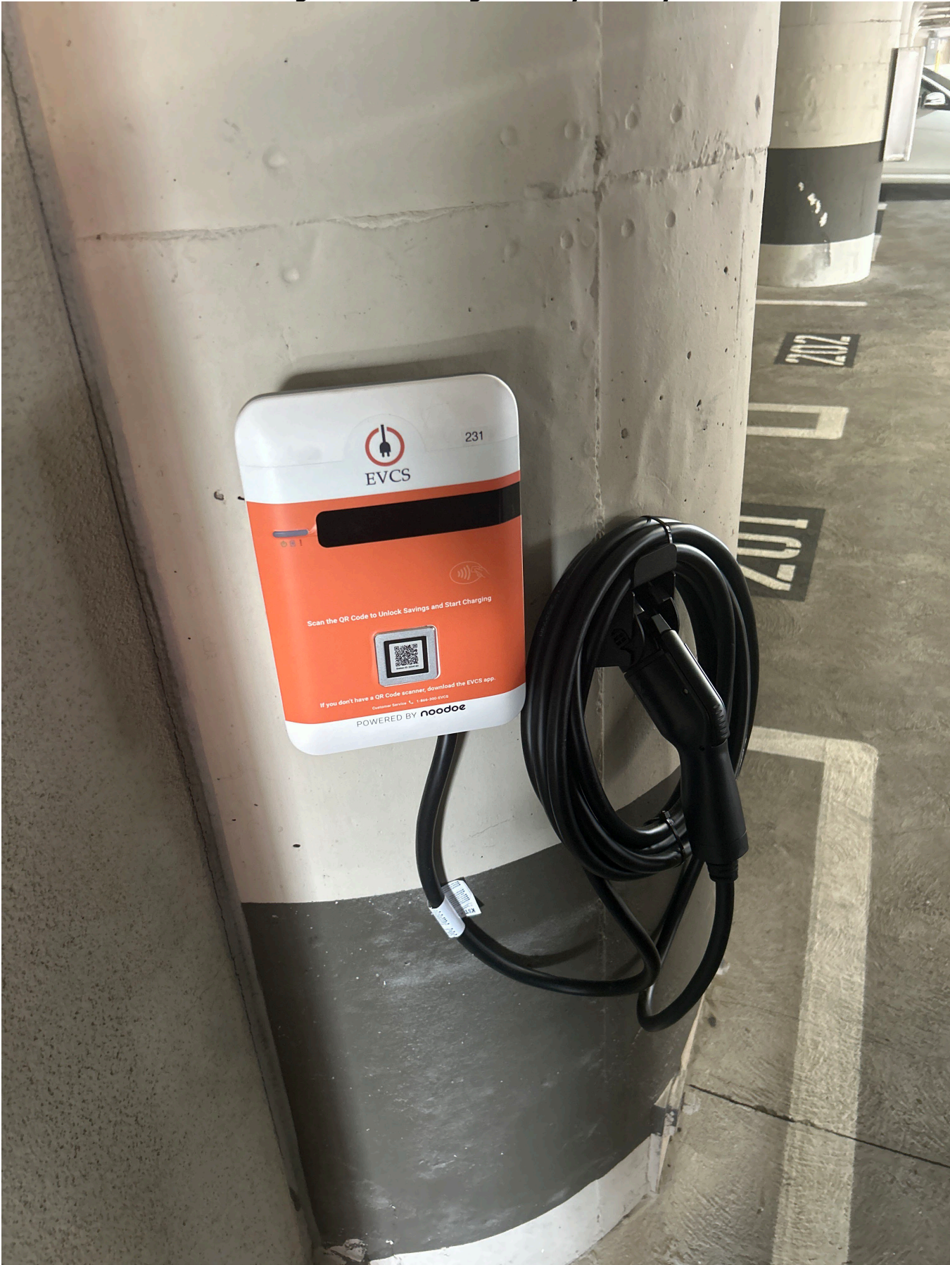
Figure 1: L2 Charger at Toy Factory
