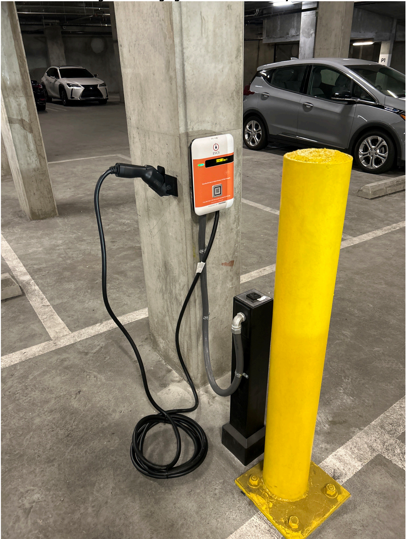
Figure 2: Charging Station at Ovelo Hollywood
