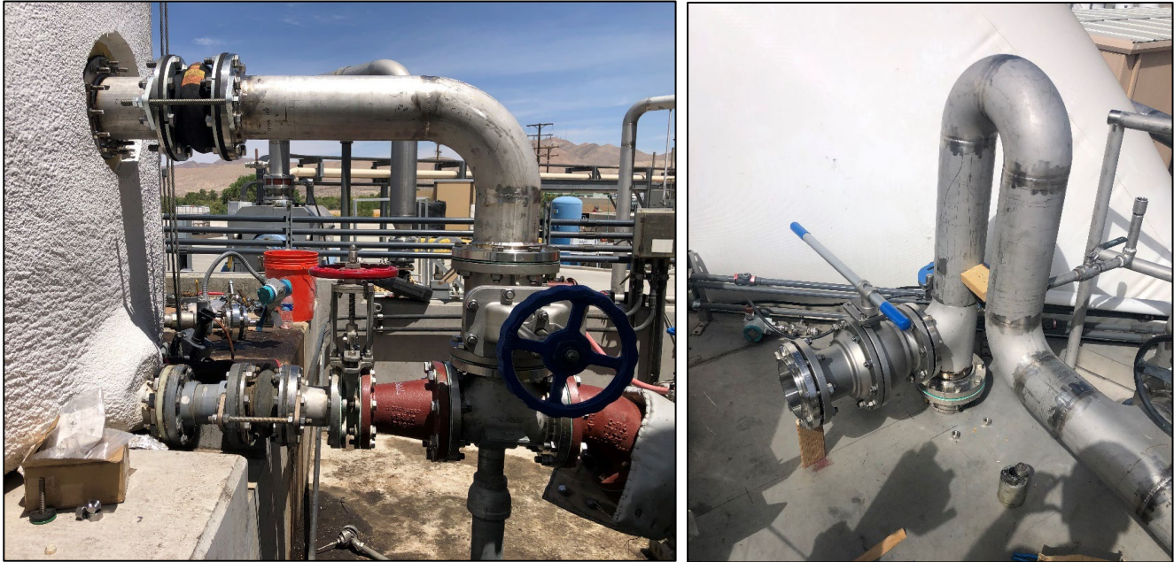
Piping modification at the Food Waste Storage Tank #1 (left) and Digester #2 (right).
