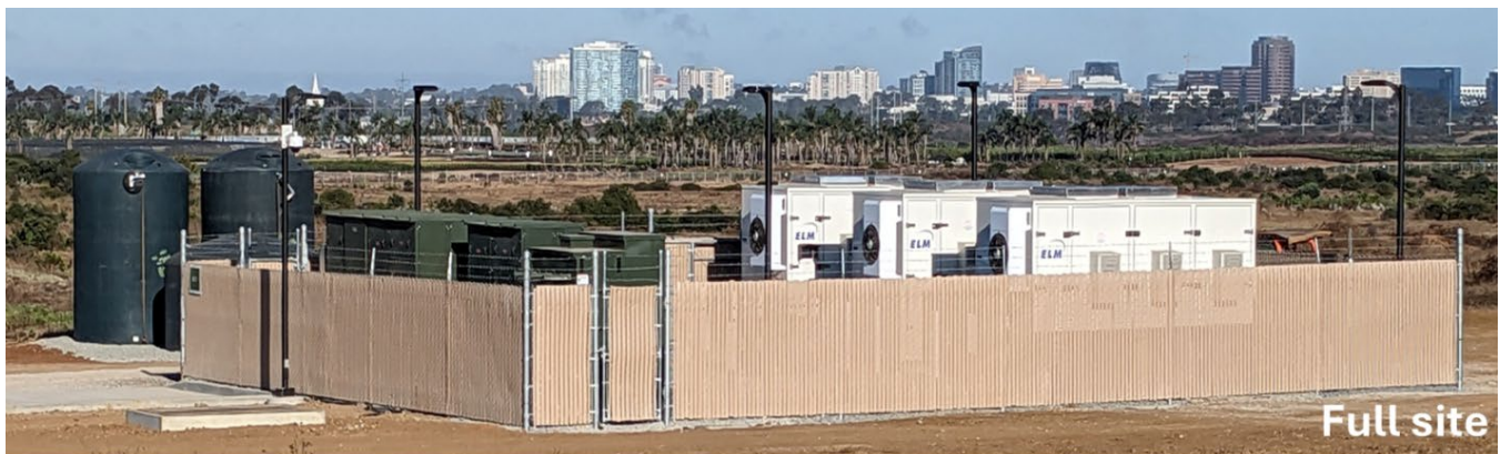
Figure 5: The Completed BESS Installation Site
