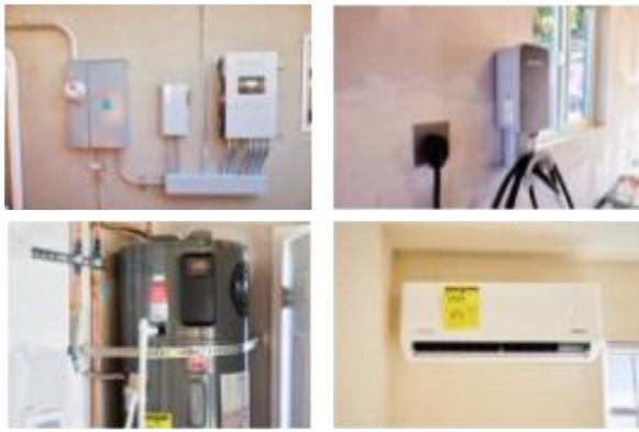
Electrification technologies installed in a VPP home
