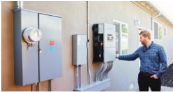
New solar system installed at participant home
