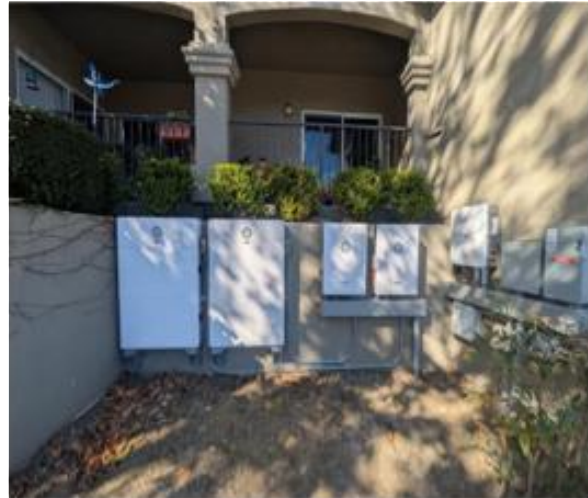
Battery storage installed at a local multifamily development
