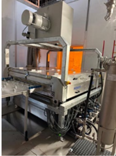
Figure 1: Newly Installed Glass Washer
