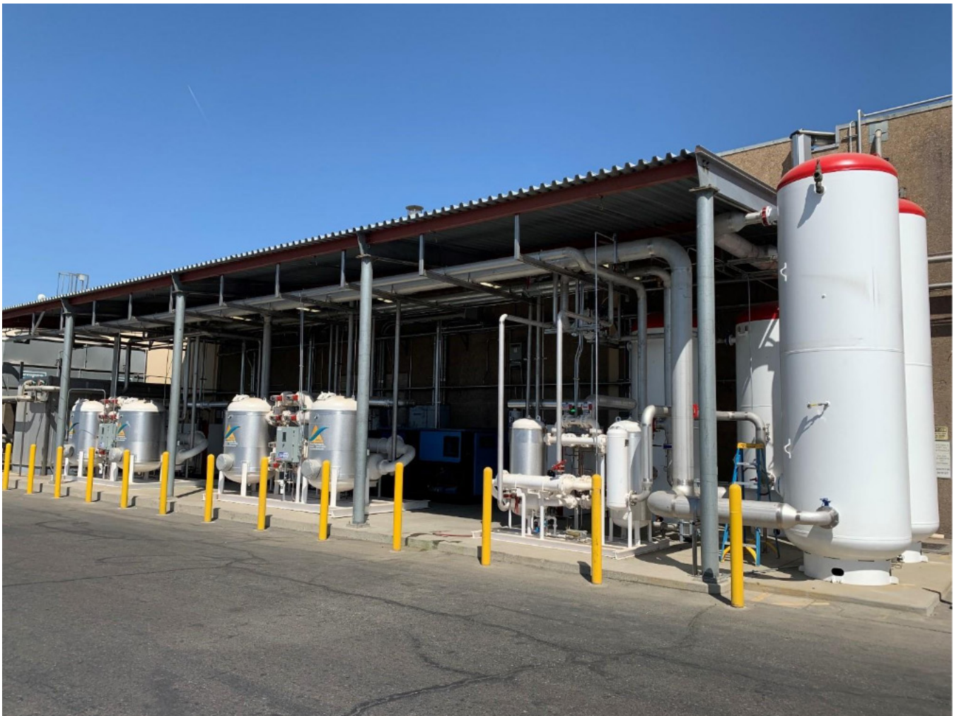
Figure 6: Overall Installed System
