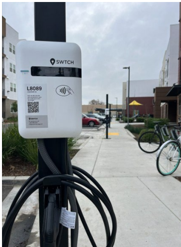
Figure 2: EV Charging Installation Photos
